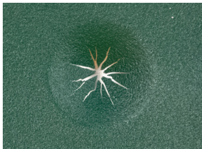
Chipping on coating layer
